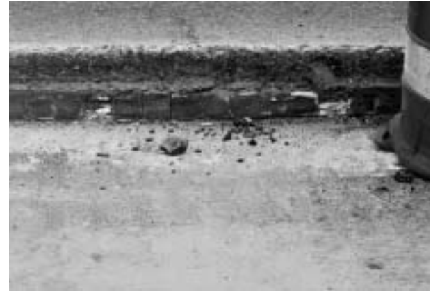
Removal of the asphalt surface and bricks leaves room for 8 inches of new, rut-resistant asphalt.
