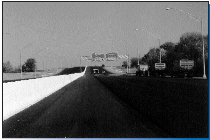
The 10.7 mile, $93 million Butler Regional Highway nears completion after only 18 months of construction
